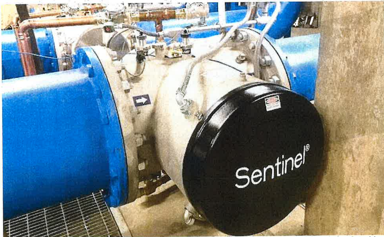
Ultraviolet (UV) reactor installed under Project WA1863. The UV system is operational and is providing additional water disinfection credit in the older 1997 Lime Softening WTP.
