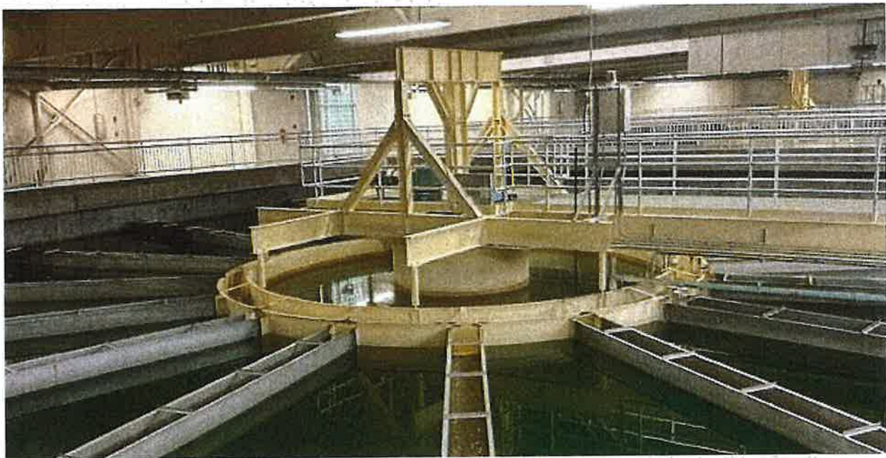
Shown is one of the secondary softening trains in the 1997 Lime Softening Water Treatment Plant. There is significant rust and corrosion on the submerged metal components. The water collection troughs were already changed to stainless steel in a project that took place over a decade ago.
