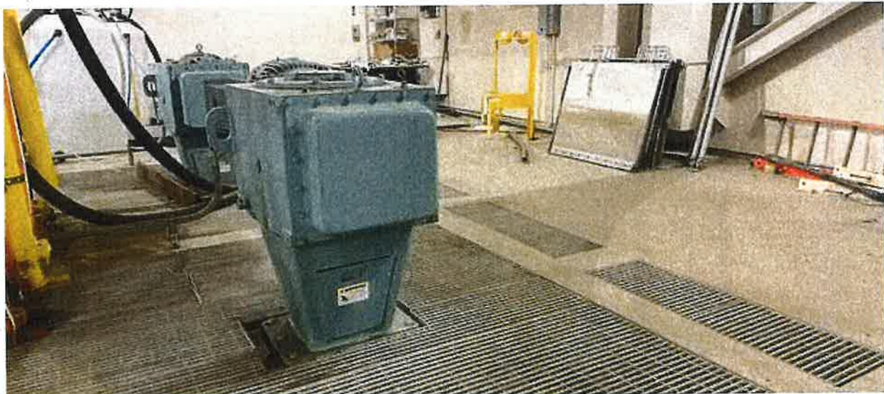
Pretreatment splitter box in the LSWTP allows for raw water flow control and was constructed to allow for WTP plant expansion from 30 million gallons per day (MDG) to 45 MGD.
