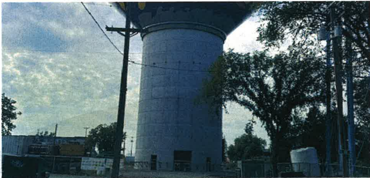
Concrete column of new water tower on which an anti-graffiti coating would be added with change order approval. The anti-graffiti coating would allow better clean-up if graffiti occurred. Graffiti has been an issue at this and other water tower sites.
