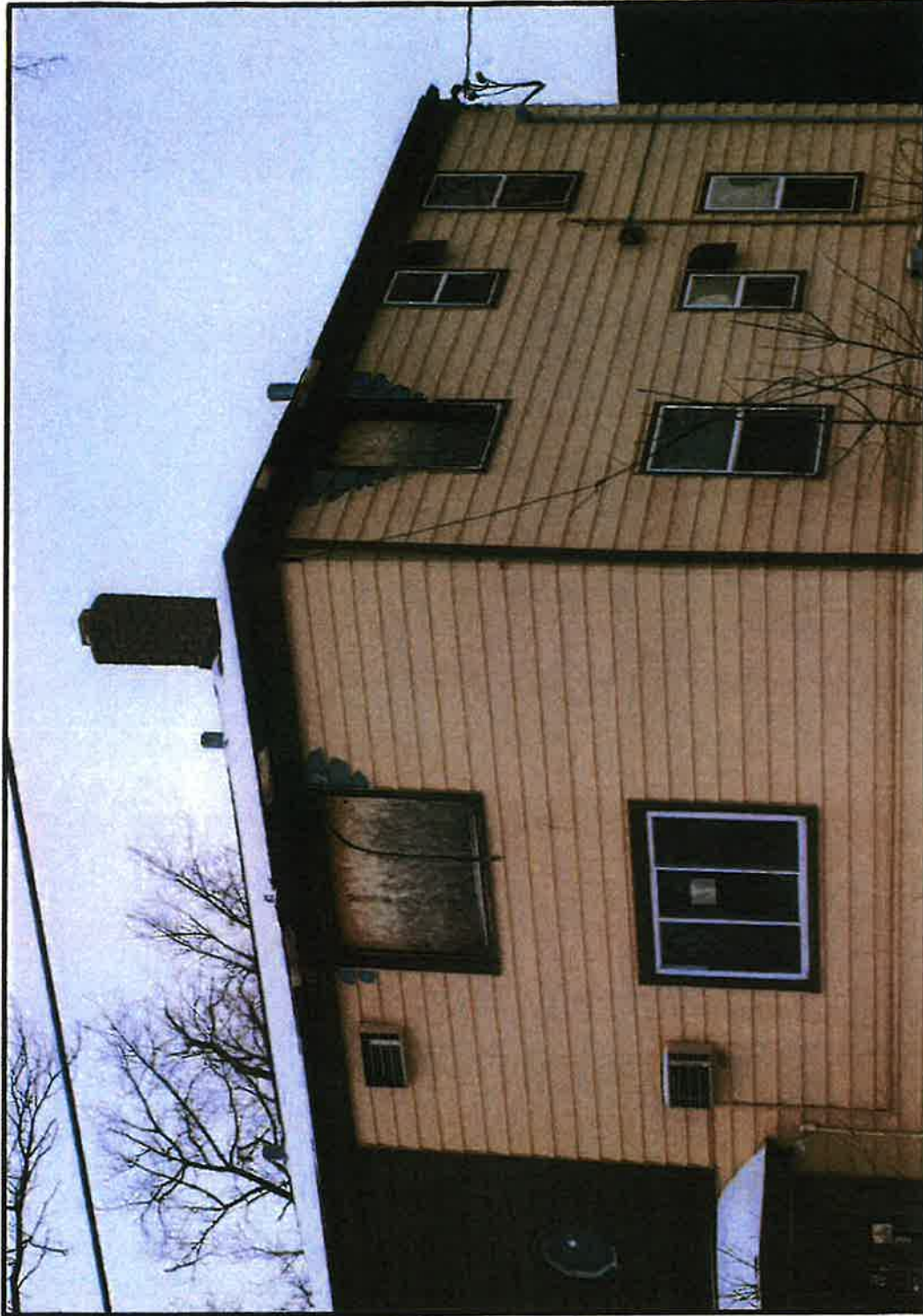
Close-up of third floor of 220 showing boarded-up windows as a result of fire damage.
