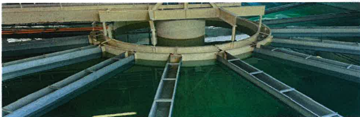
Picture of a Secondary Softening Basin in the Fargo WTP. Corrosion is visible both above and below that water surface.
