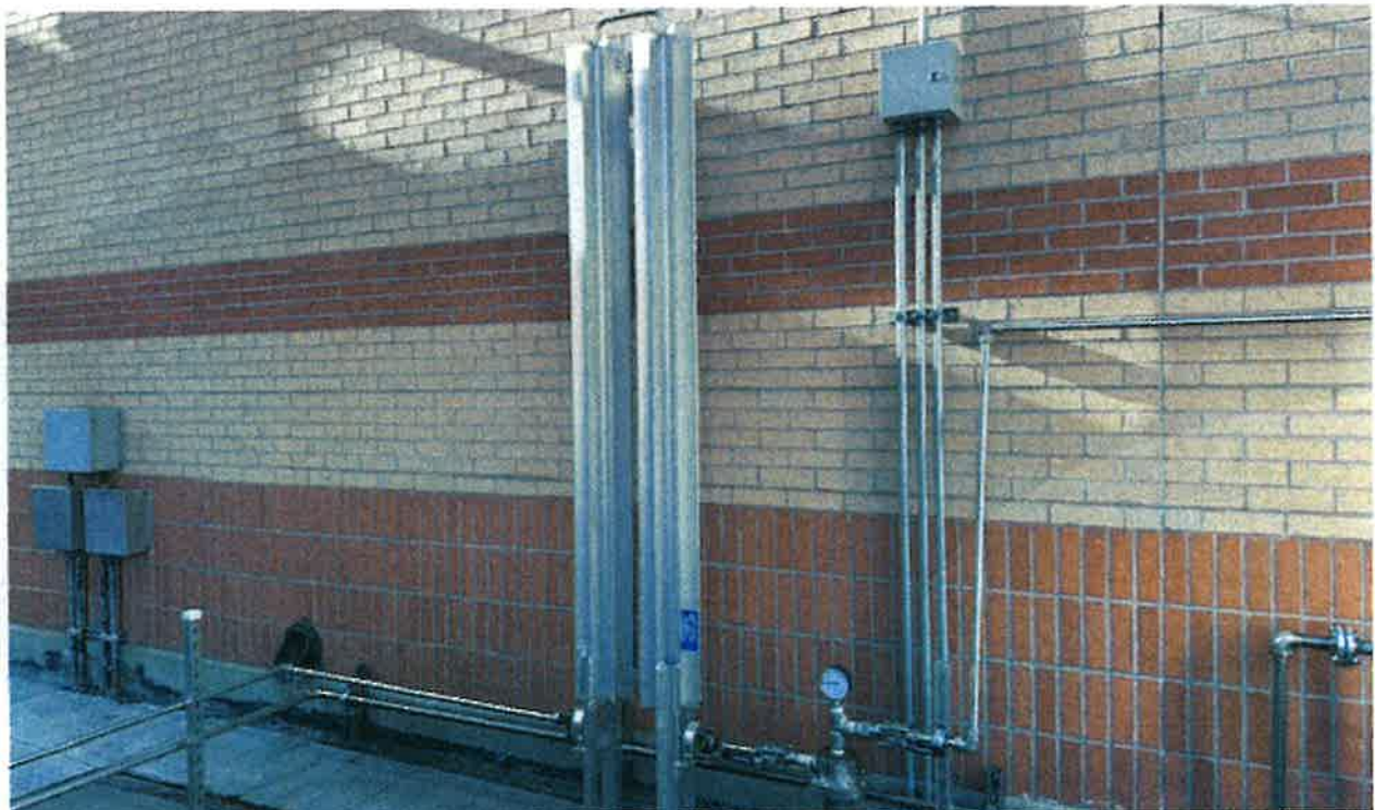
Pictured is some of piping and equipment installed by a specialty contractor to vent Liquid Oxygen (LOX) tank pressure for use in ozone generation (treatment cost efficiency). Apex needs to generate drawings for the North Dakota Department of Environmental Quality (NDDEQ).
