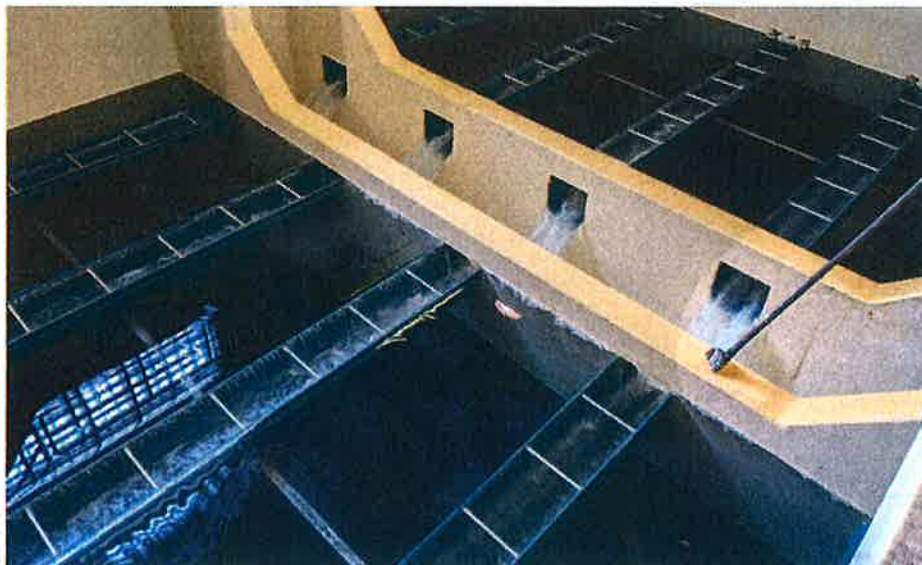
Existing Lime Softening WTP Filters
