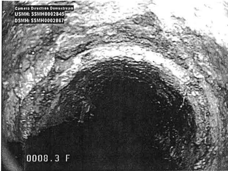
North Failure – CIP Joint Separation
