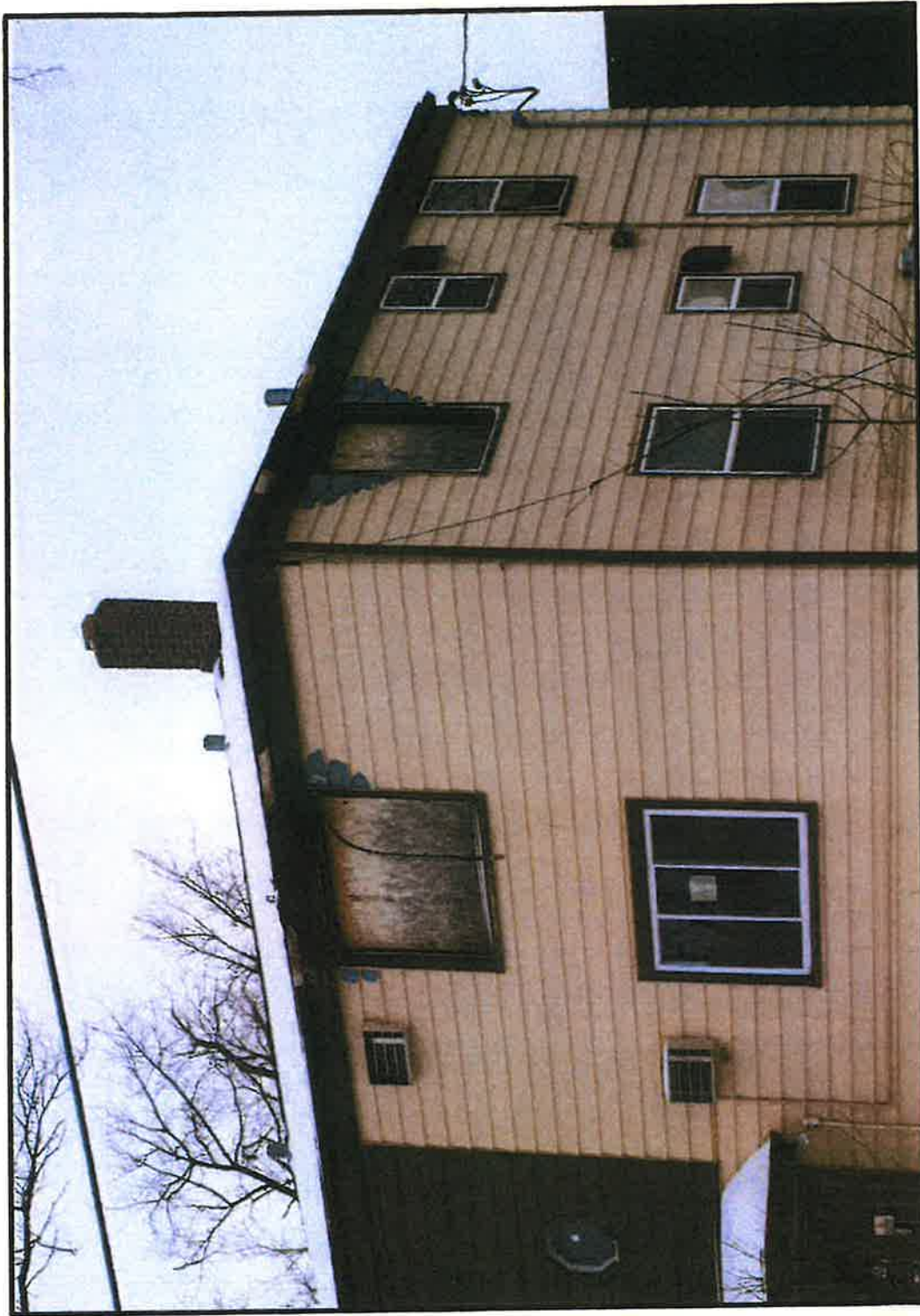
Close-up of third floor of 220 showing boarded-up windows as a result of fire damage.
