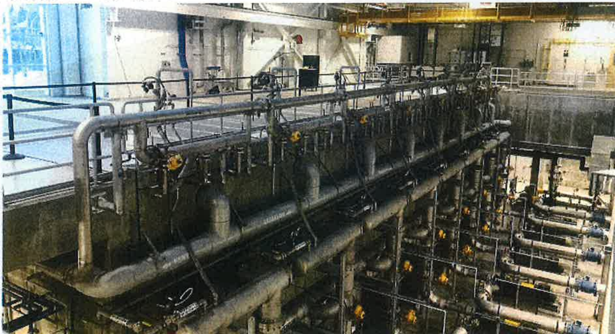
Picture of the valves and piping for the Suez Microfiltration/Ultrafiltration (MF/UF) membrane process. This process removes particles from water prior to Reverse Osmosis. In addition, the MF/UF process attains significant EPA credit toward pathogen removal.
