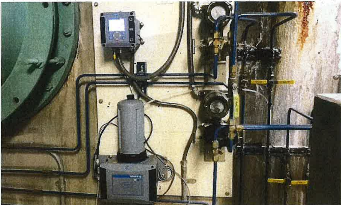
Installation of new turbidity (water clarity) analyzer in the 1997 WTP, completed by Sun Electric, Inc. under the 2022 Electrical Services Agreement. Turbidity measurements regulated by the EPA.
