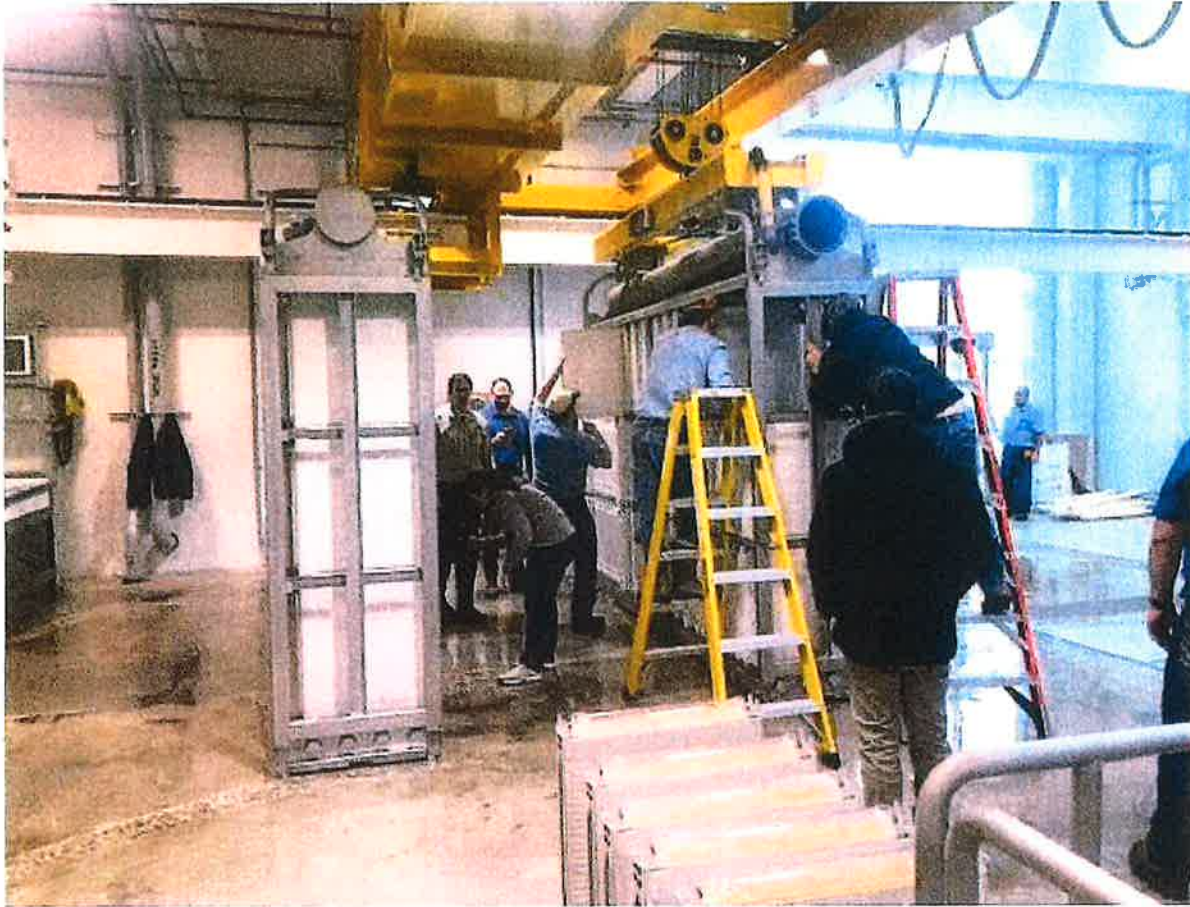
The above picture shows two Suez Ultrafiltration (UF) cassettes. Water Utility personnel and consultants were performing a UF membrane module addition project in April, 2022.
