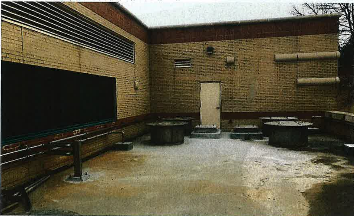
Picture on top of ozone chambers with safety features installed that will provide fall protection and allow for safe work in a single contact chamber with the other one in operation
