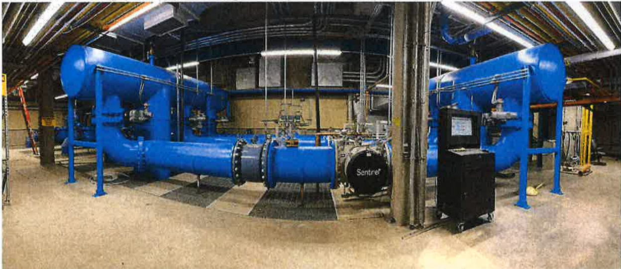
Picture of Ultraviolet (UV) Reactors and flow meters installed with Project WA1863. This is a completely new disinfection system for the 1997 Lime Softening Water Treatment Plant. (Picture by Marisha Lunde)
