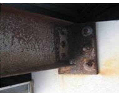
Figure 11 - Structural Steel & Rust Scaling
