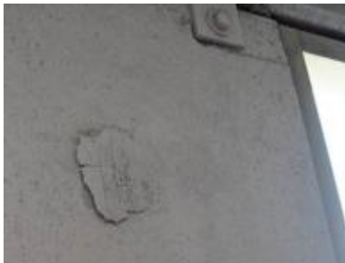
Figure 1- Failing Concrete Patch
