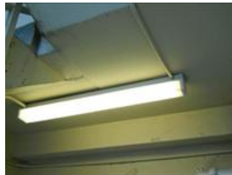
Figure 22 – Fluorescent Light Fixture
