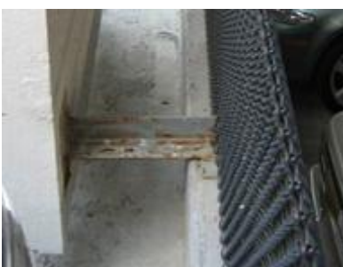
Figure 10 - Structural Steel Rusting
