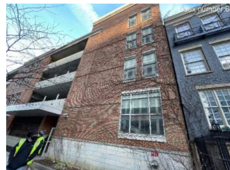
Figure 36 - Dead Vines to be Removed from Facade
