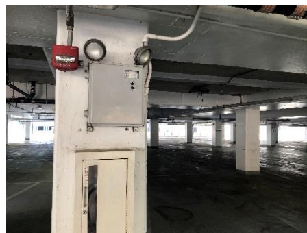
Figure 28 – Typical Smoke Detector
