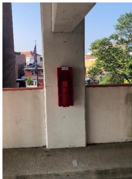
Figure 27 - Typical Fire Extinguisher
