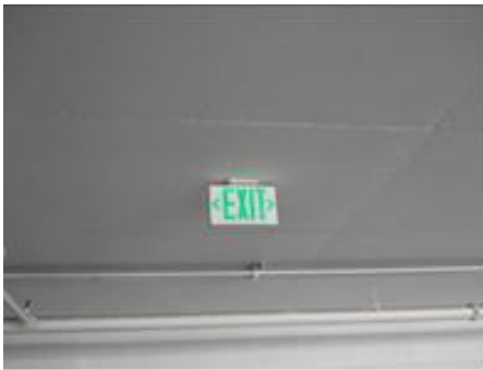
Figure 23 - Typical Lit Exit Sign
