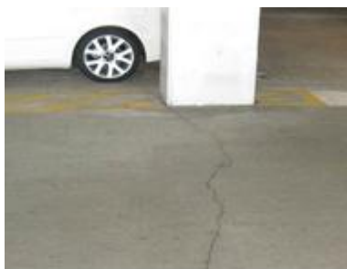
Figure 5 – Medium Crack, 0.01” to 1/32” Width
