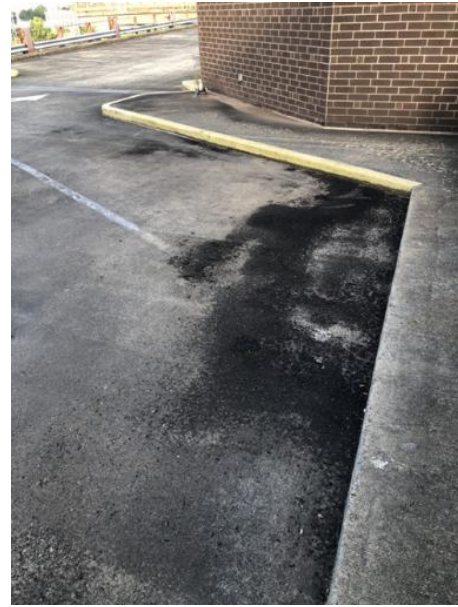
Figure 18 – Dirt / Stains on Driving Surface
