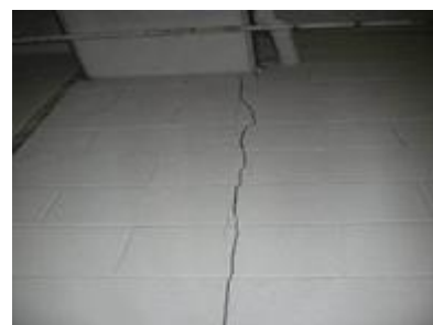
Figure 6 – Wide Crack, greater than 1/32” Width
