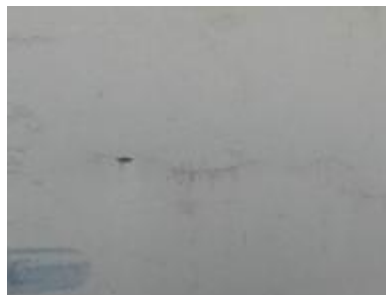
Figure 4 – Fine Crack, 0.1” Width or Less
