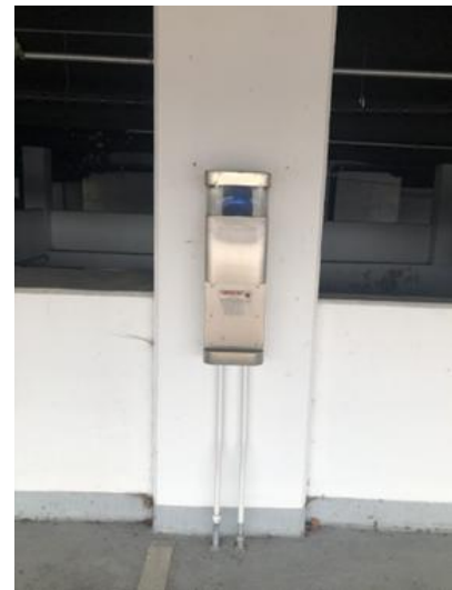
Figure 33 - Typical Emergency Call Station
