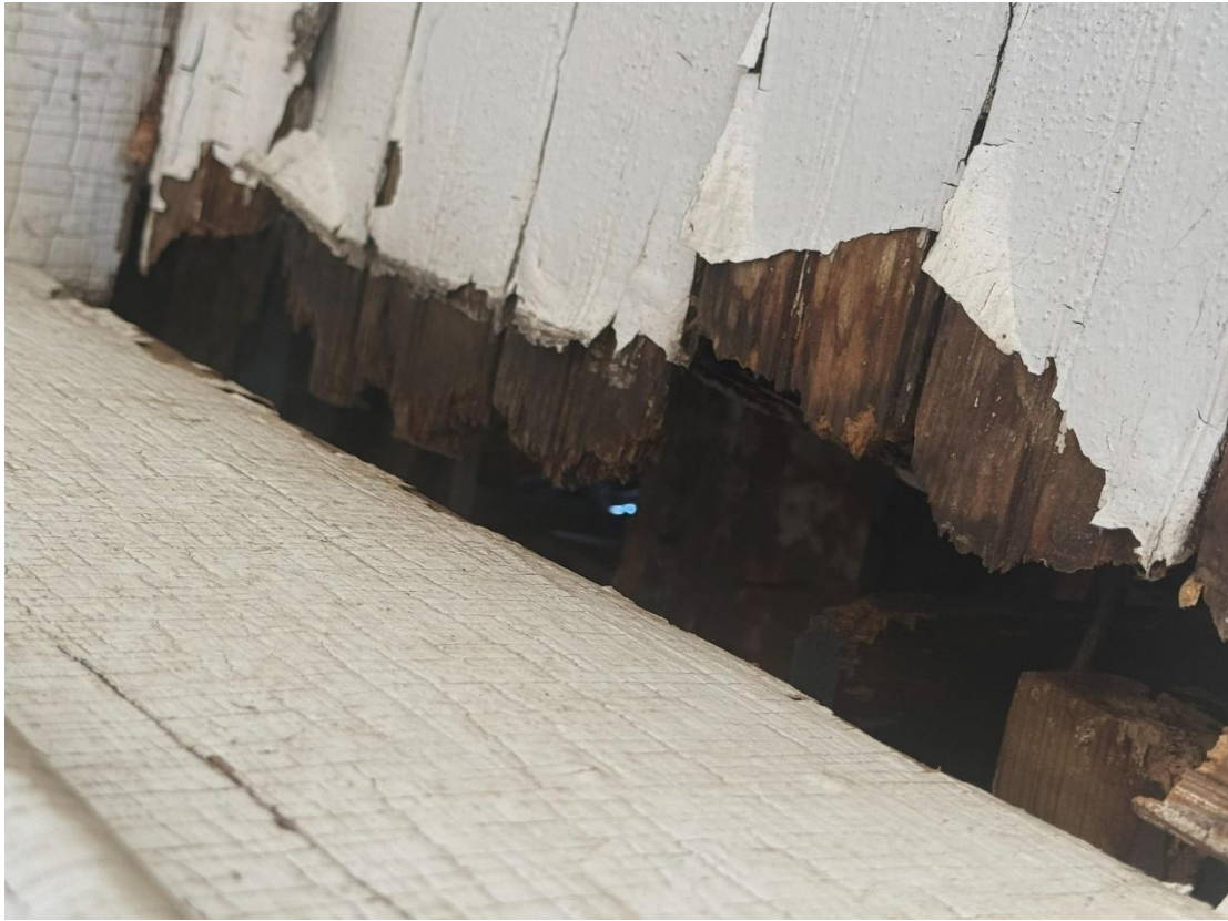
This picture shows the rot in the ceiling under the upper level deck. This rot goes into the structural joists of the upper level.
