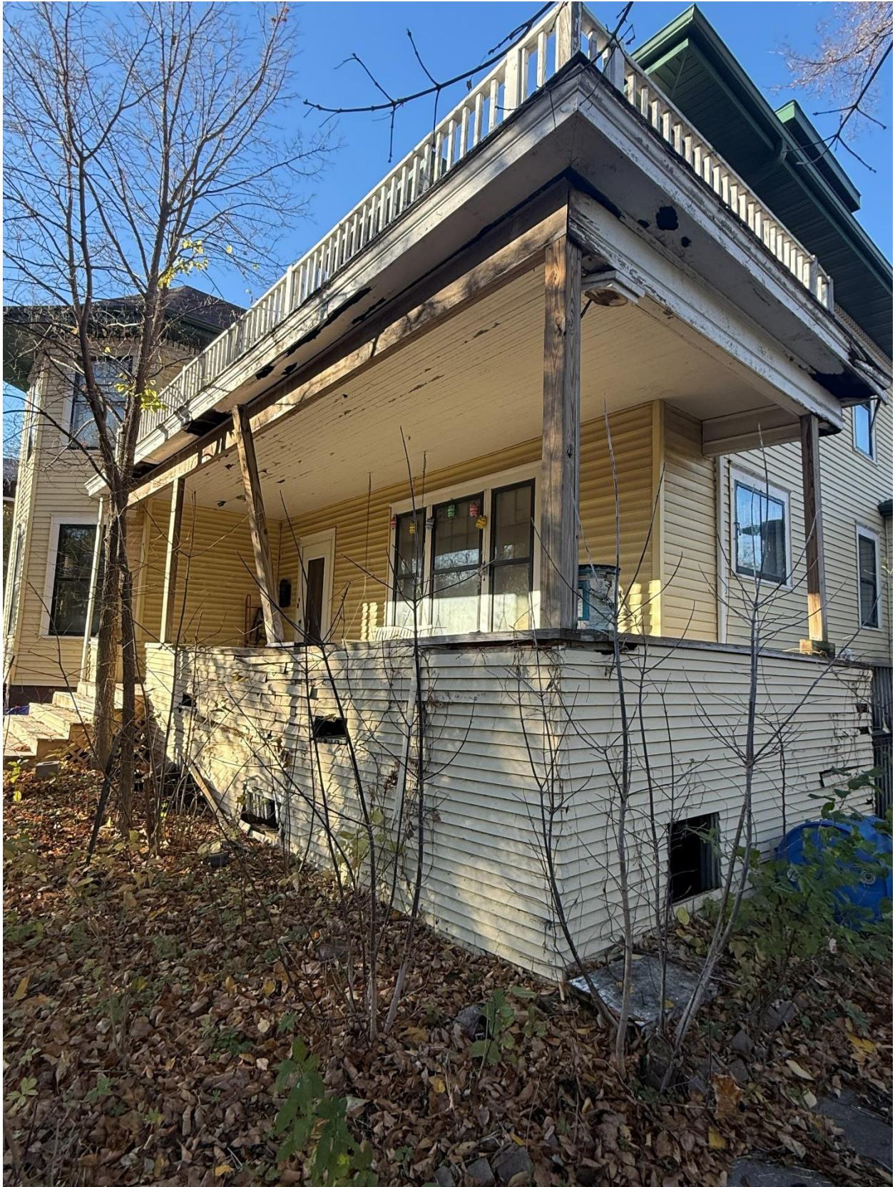
This picture shows the support columns falling out and the upper support beams are not exterior rated materials.
