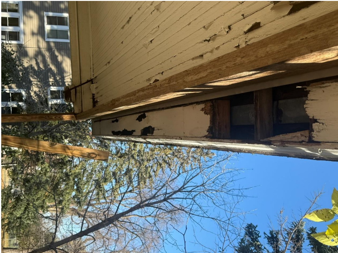
This picture shows the materials falling off the ceiling and eaves on the upper level. This is rotten beyond repair.
