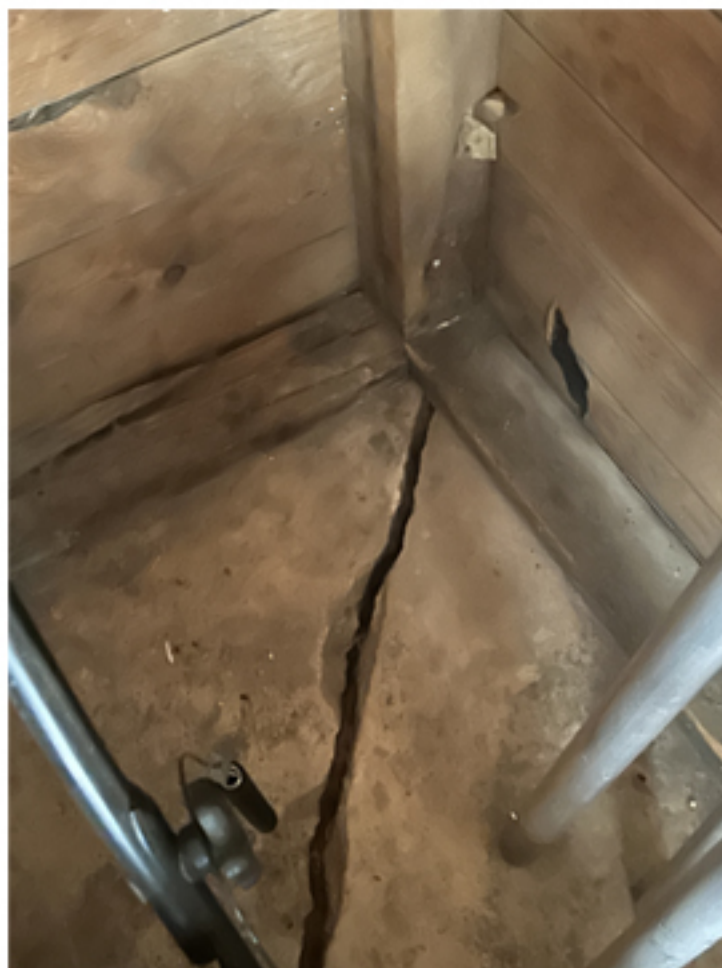
Slab & Sill Plate Cracking
