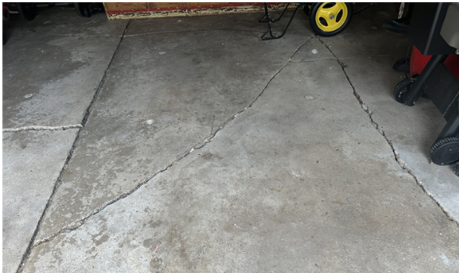
Interior Slab Cracking
