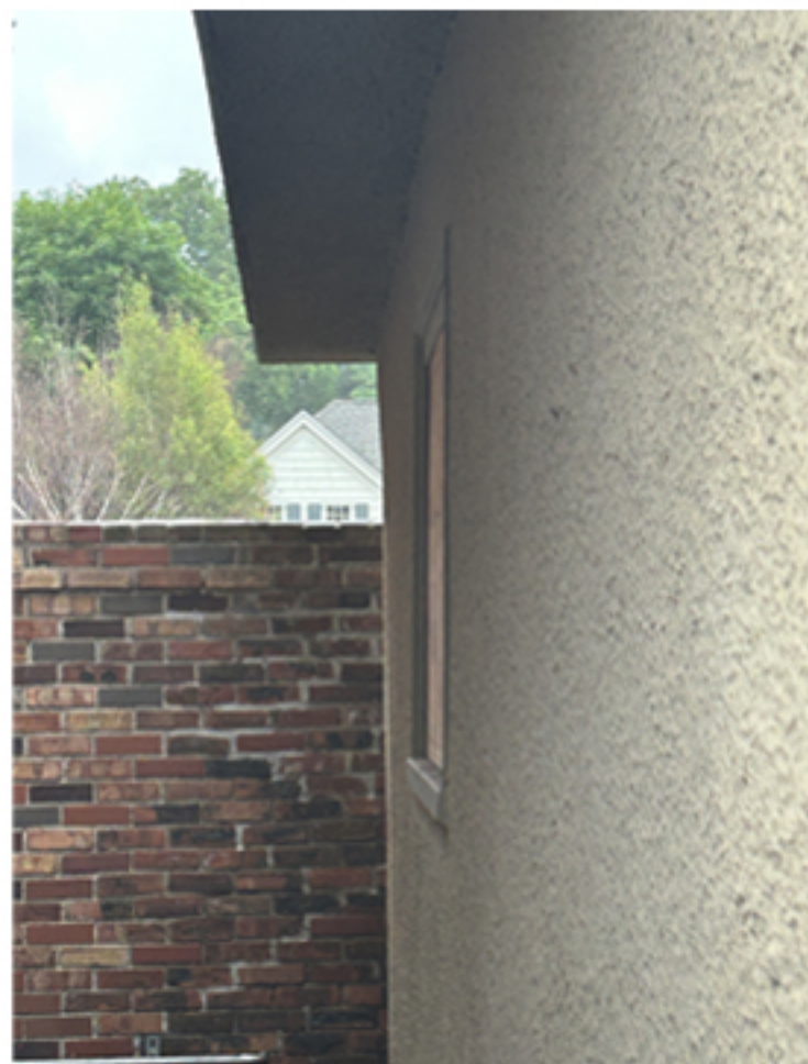
Exterior View - Bowing Wall
