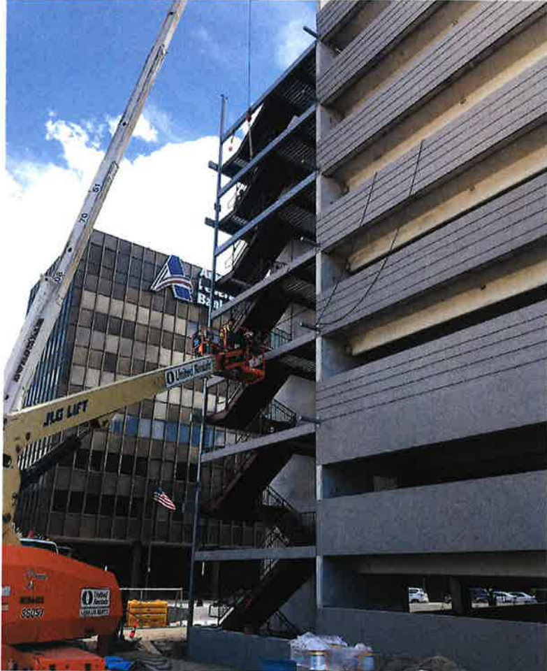
Photo 3 – Northeast stair tower metal stair installation nears topping out. Mobile erection crane working from 3 rd Avenue North
