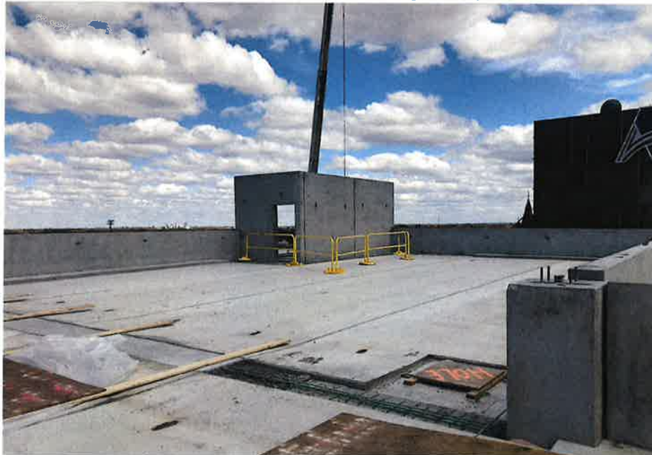
Photo 2 – Parking Garage precast erection complete. Looking north east at north stair tower. Curb and concrete wash installation just beginning from top down.
